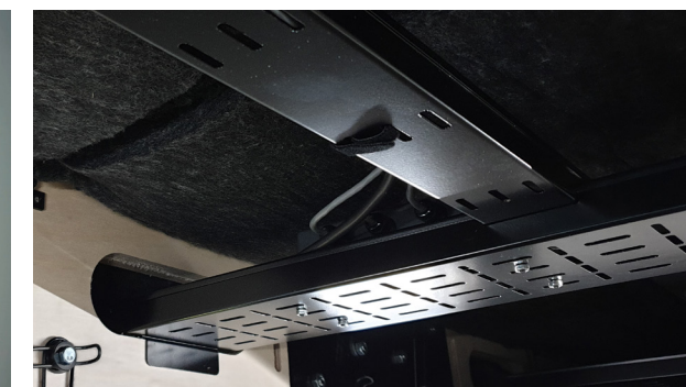
Cable-management within ceiling
