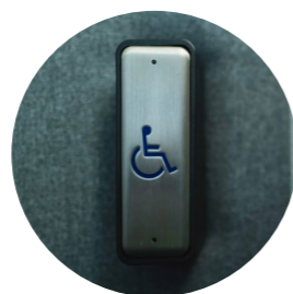
Auto Door opener inside & outside on DDA booth
